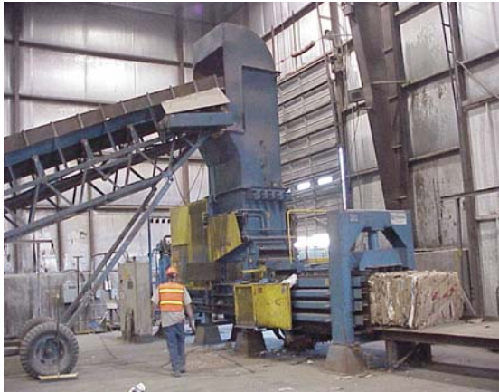
BAILER FOR RECYCLABLE REFUSE COLLECTED IN THE TRANSFER STATION
